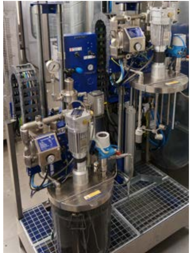
supply center diaphragm pumps agitator, level control
